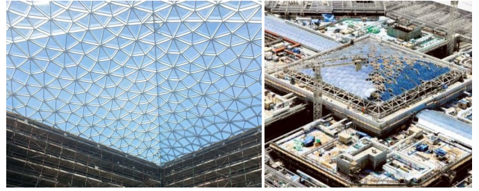
Figure 43: Yas Mall, Abu Dhabi: Gridshell with ornamental polyhedral pattern. Image at left: Stutzki Engineering Newsletter. Image at right, showing construction: Aldar.
